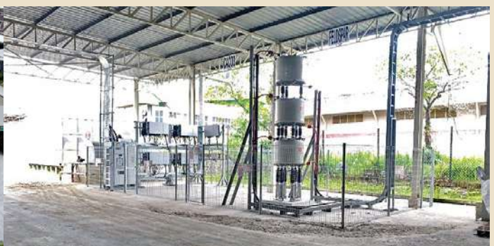
Figure 2: Meter and Breaker Panel, Inverter Station and Fault Current Limiting Reactor (FCLR) at KHCS Plant 1
